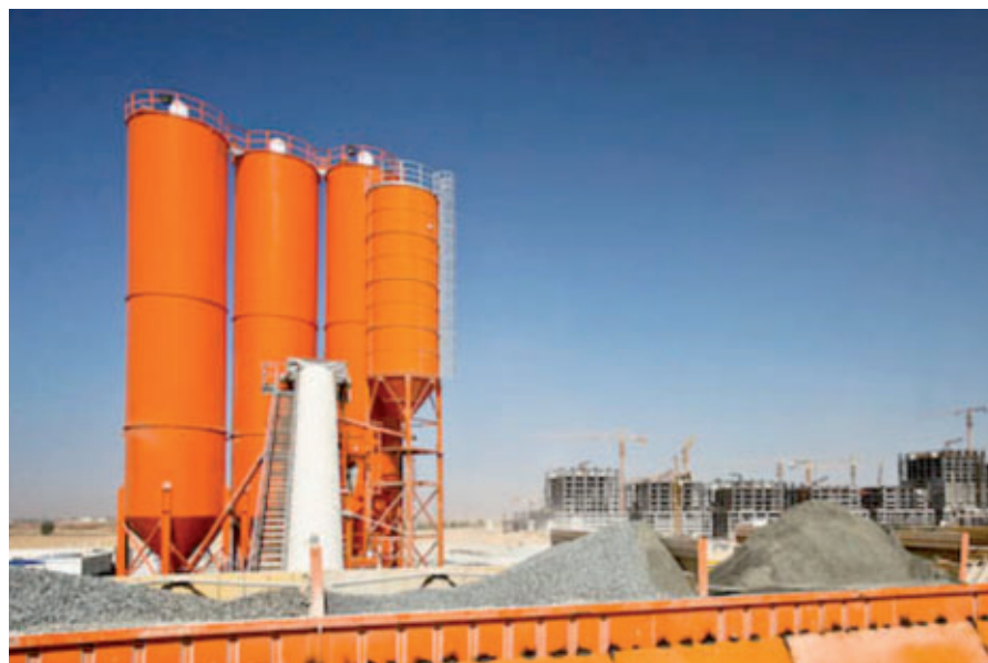
Each mixing plant is equipped with a total of 3 cement silos and a microsilica silo
